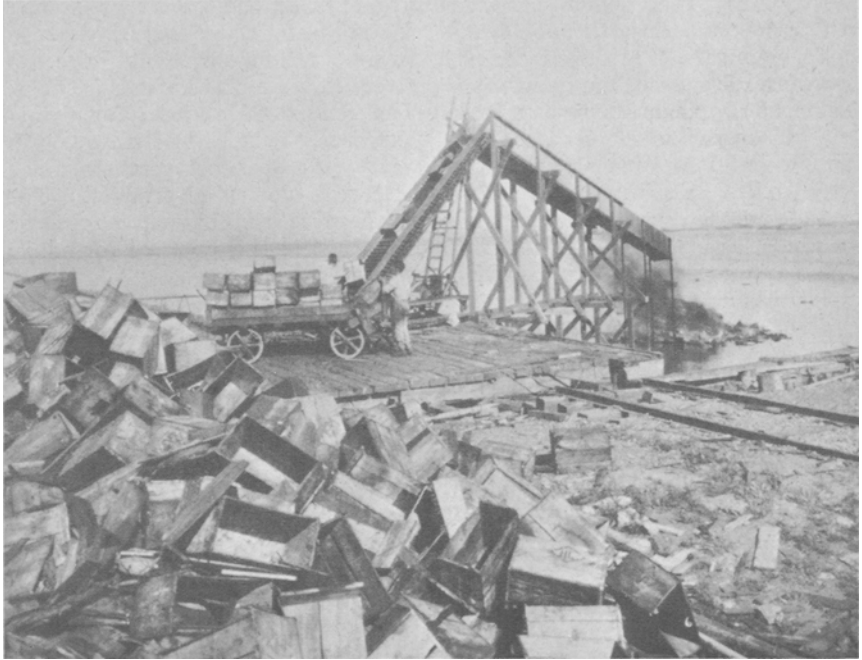
Near view of one of many conveyors for moving and burning oil-soaked wooden cases
